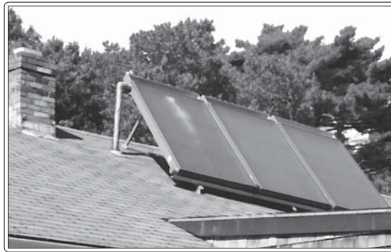
This solar water heater has been on Bob Gardé's roof for twenty years
